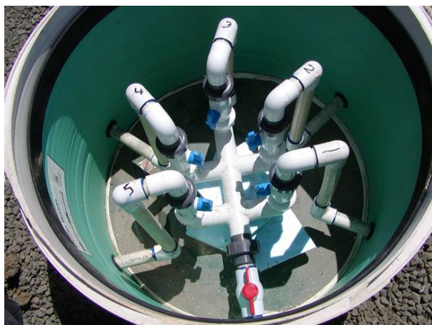
An accessible and well-marked hydrosplitter. Photo courtesy of Brian Rabe, Cascade Earth Sciences
