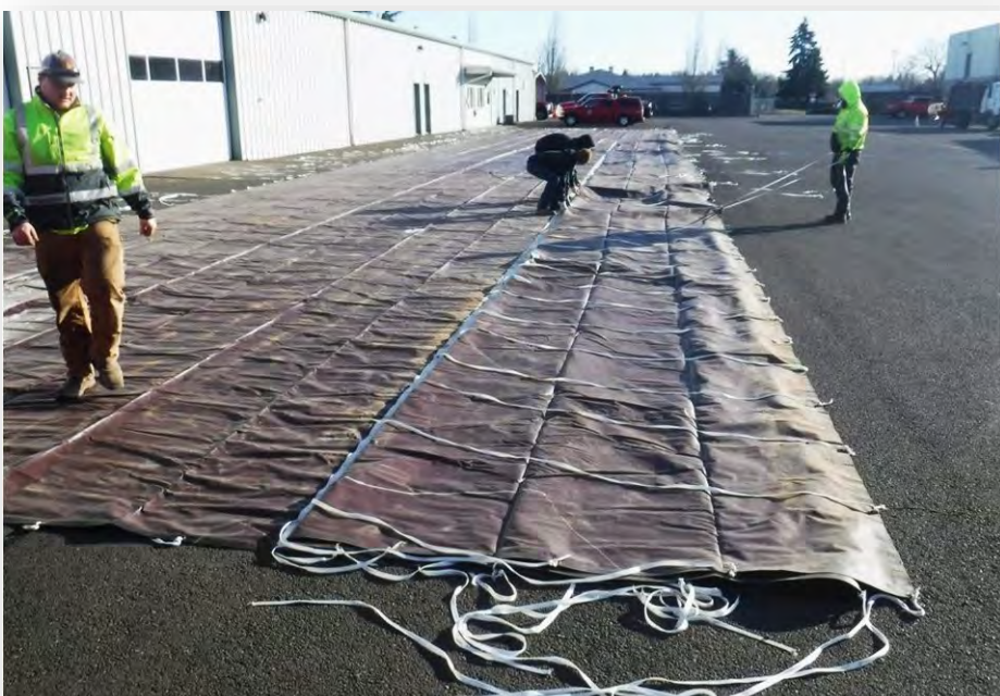
Linn County Bridge Crew members Layne Newman, left, Marcus Jones, center front, Tyler Miller, center rear, and Rusty Thorpe, right. Photo: Rich Gilbert.
