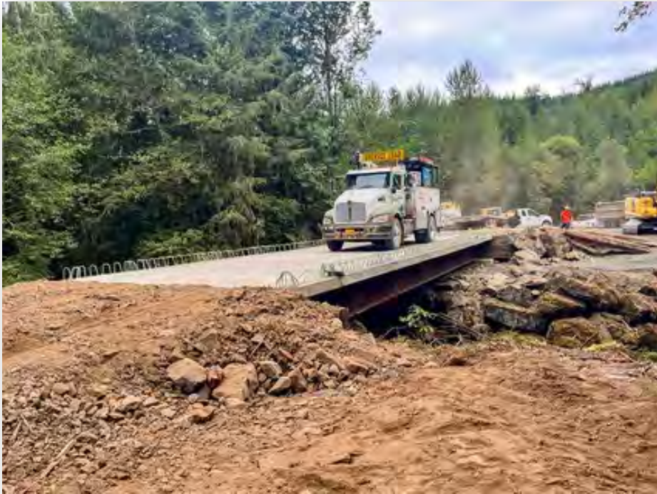
Having a bridge pre-made allowed workers to install it in record time to service the Wiley Creek Fire west of Sweet Home.
